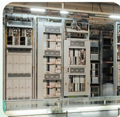
D10 Electric Switching System
